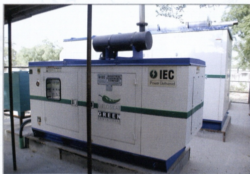
Diesel Generating Sets
